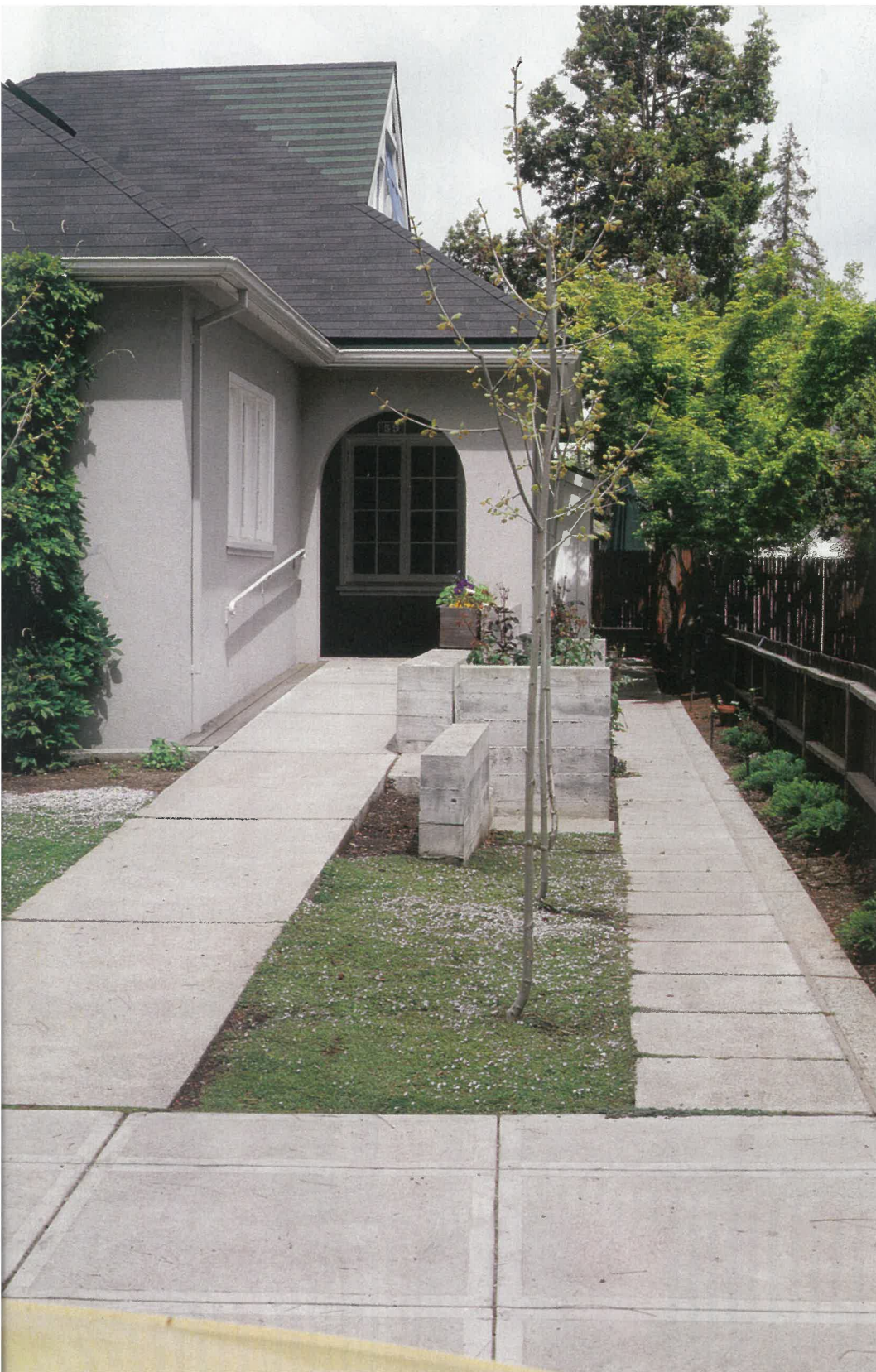
Streetside. The new path to the front door rises on an incline, bearing largely on fill brought in to raise the grade gently. Note the green stripes in the dormer—they delineate the new construction from the original roof.
